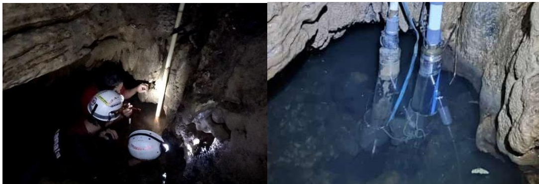
Picture 2 & 3, the installation of the water lifting pump and the pump system installed in Keceme Cave, Girisekar, Panggang, Gunungkidul, Yogyakarta
